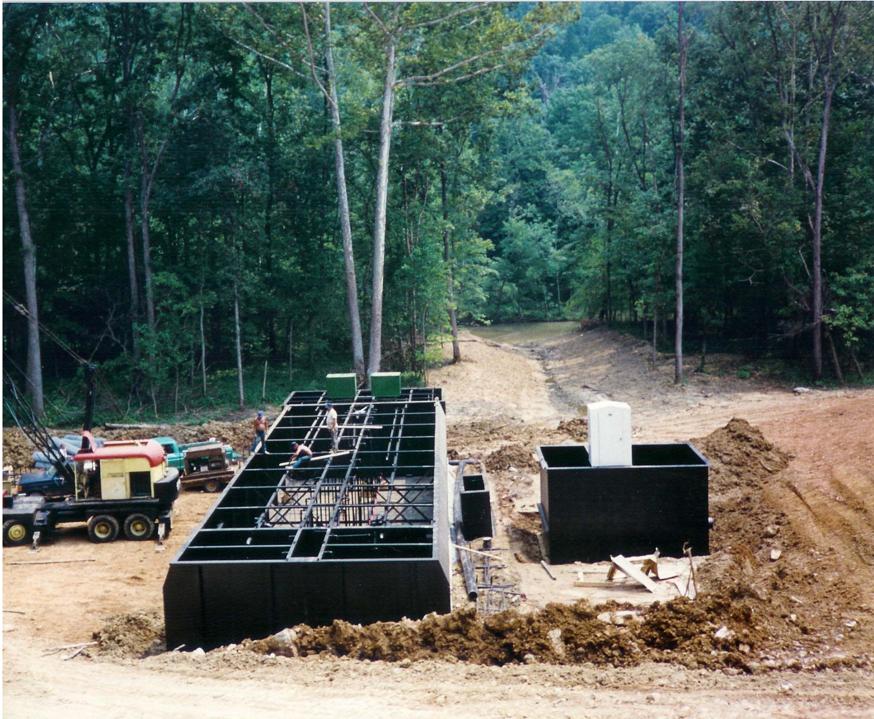
Paramount Estates, 120,000 gpd Plant
