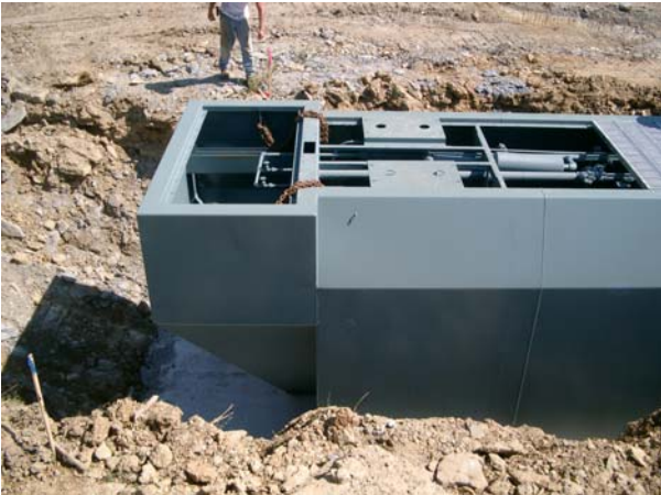
Figure 3) Clarifier hopper end of WWTP
