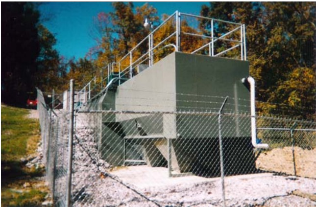
Figure 3) 30,000 gpd WWTP with Integral Chlorine Contact Tank
