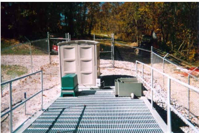
Figure 5) Chlorine Shed, Flow Control Box, Flow Equalization Blower
