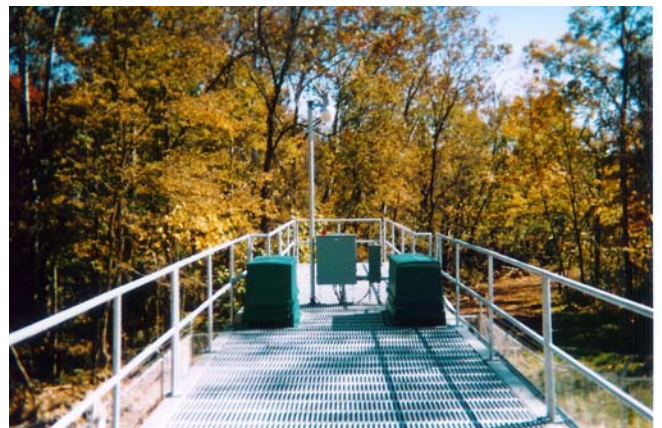
Figure 5) Full Grating, Perimeter Hand Rail, Main Blowers, and Control Panel
