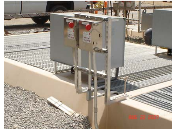
Fig. 4) Treatment plant blowers with electrical disconnect in foreground
