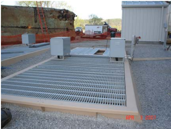
Fig. 3) Flow Equalization Tank and Treatment Plant
