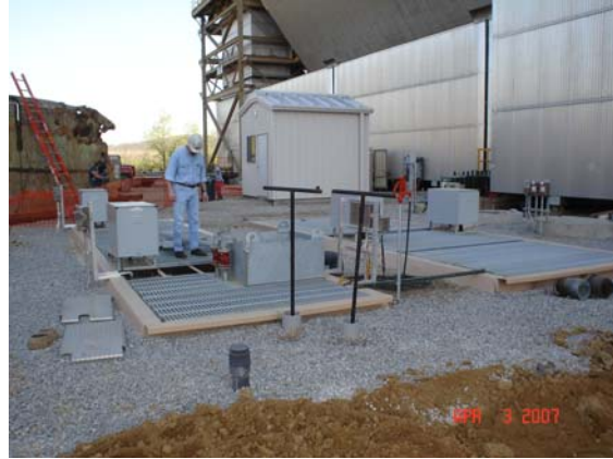
Fig. 2) Flow Equalization Tank (left) and Treatment Plant (right)
