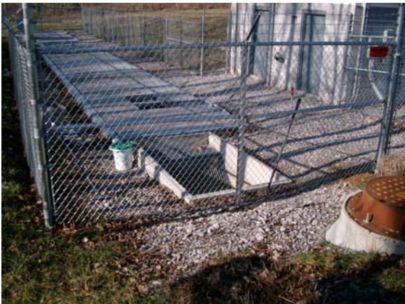
Figure 3) 30,000 gpd WWTP with Concrete Inlet Bar Screen Box
